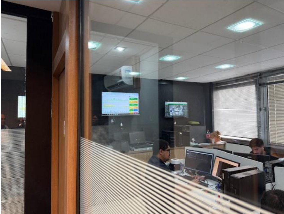
Figura 4 - Data Center e Service Desk
