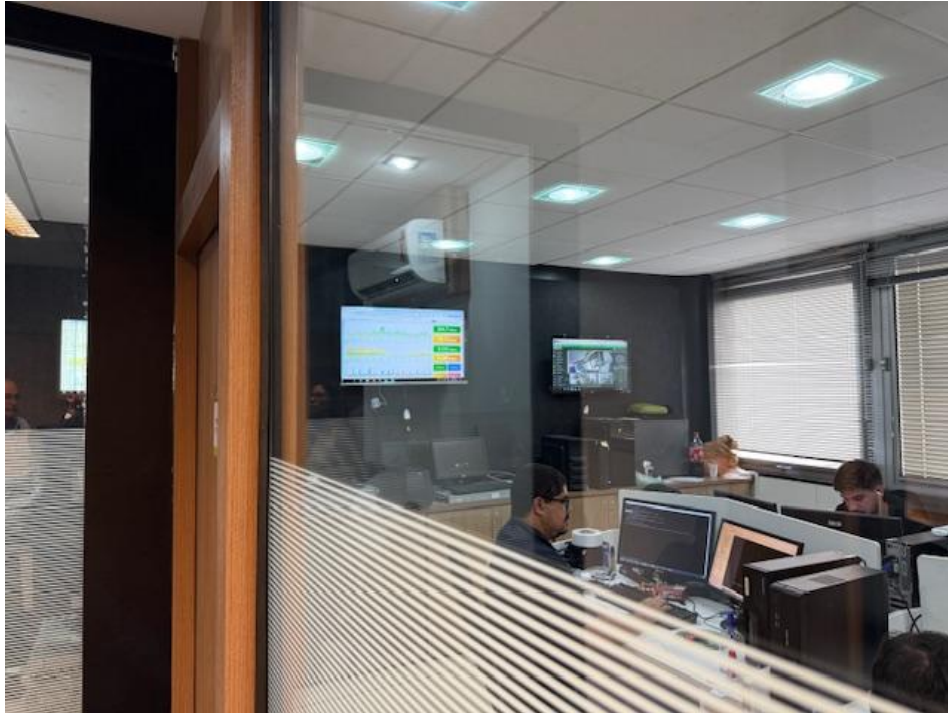
Figura 4 - Data Center e Service Desk
